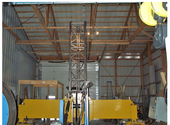
The Deep Ice Sheet Coring tower (under construction) that will provide the infrastructure to lower the drill down the borehole.
